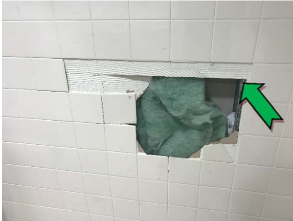
Photo 1. Interior, level 1, male and female toilets, wall lining – non asbestos-containing fibre cement sheeting.
