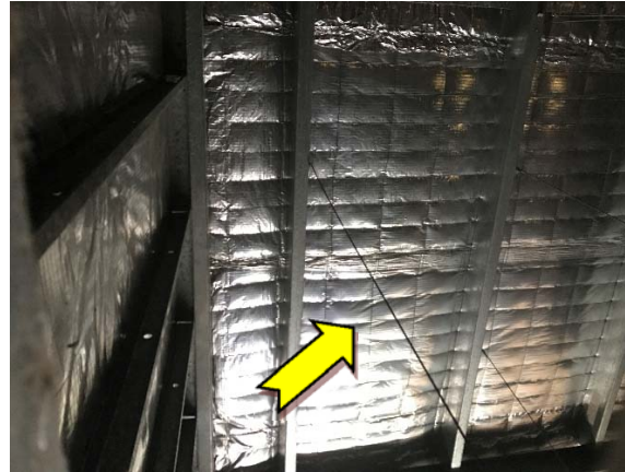
Photo 2. Interior, throughout, above suspended ceiling, sarking insulation – suspected SMF insulation.
